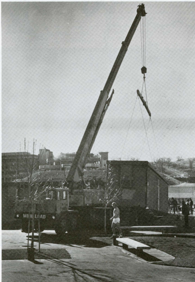
An era (the "Stalag 13" period) is ending at COC as portable structures that served as classrooms and office for several years are moved out. In background are new Bonelli Center and the Laboratory building, the latter still under construction.
