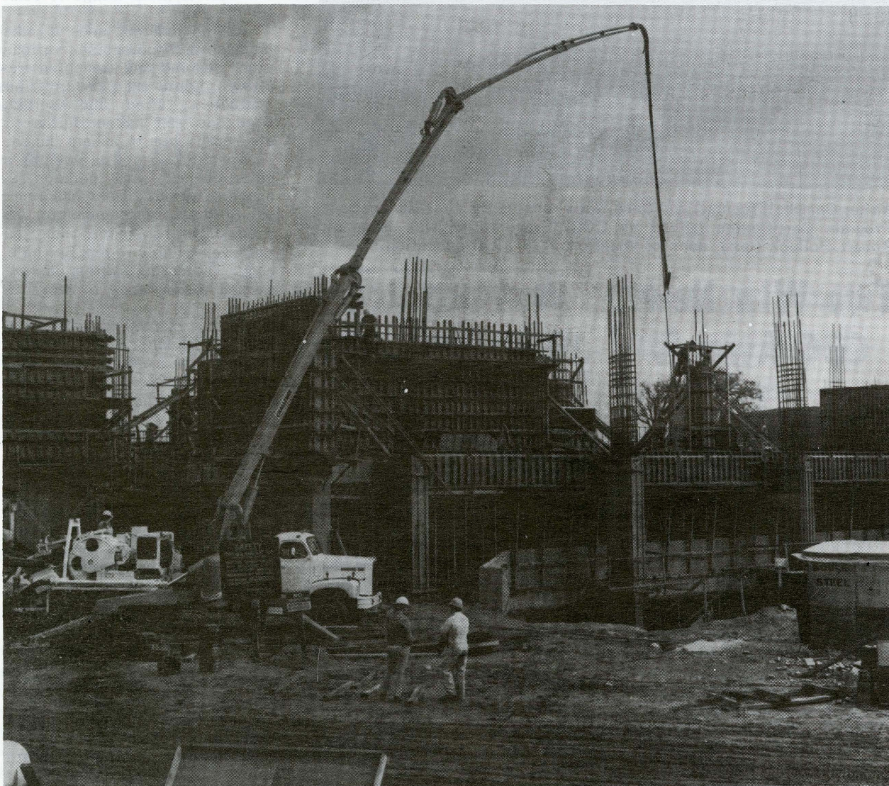
A hydraulic concrete pump with a 110-foot boom, reputedly the only one of its kind, is pumping concrete into the third-floor columns and walls of the William G. Bonelli Instructional Resource Center under construction on the south campus. The pump lifts concrete through the boom at the rate of 60 cubic yards an hour, saving many man-hours over more conventional systems. Engineers are hopeful of pouring the last floor in the four-story structure by the end of April.
