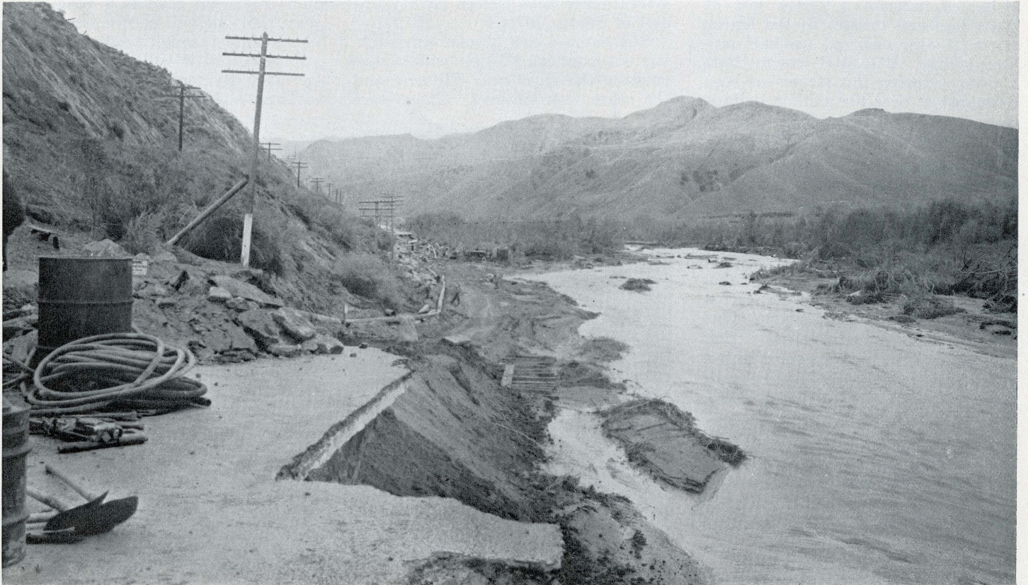
This picture vividly reveals damage wrought by Santa Clara River floods on Ventura-Castaic lateral highway between Piru and Los Angeles County line in Ventura County.
