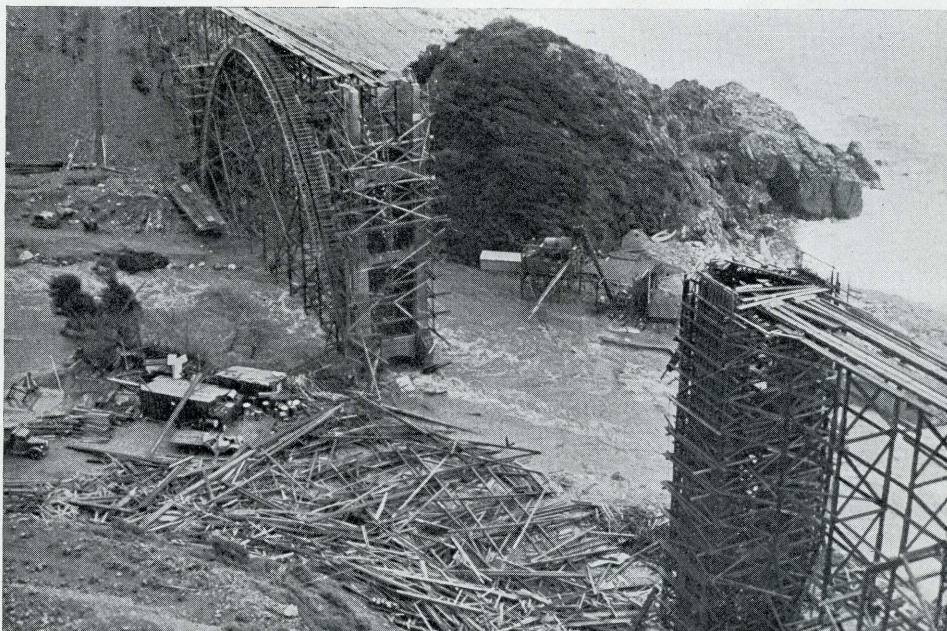
Bridge under construction across Big Creek on the San Simeon-Carmel coast highway in Monterey County. Concrete piers withstood flood waters but high winds blew down falsework of one arch.
