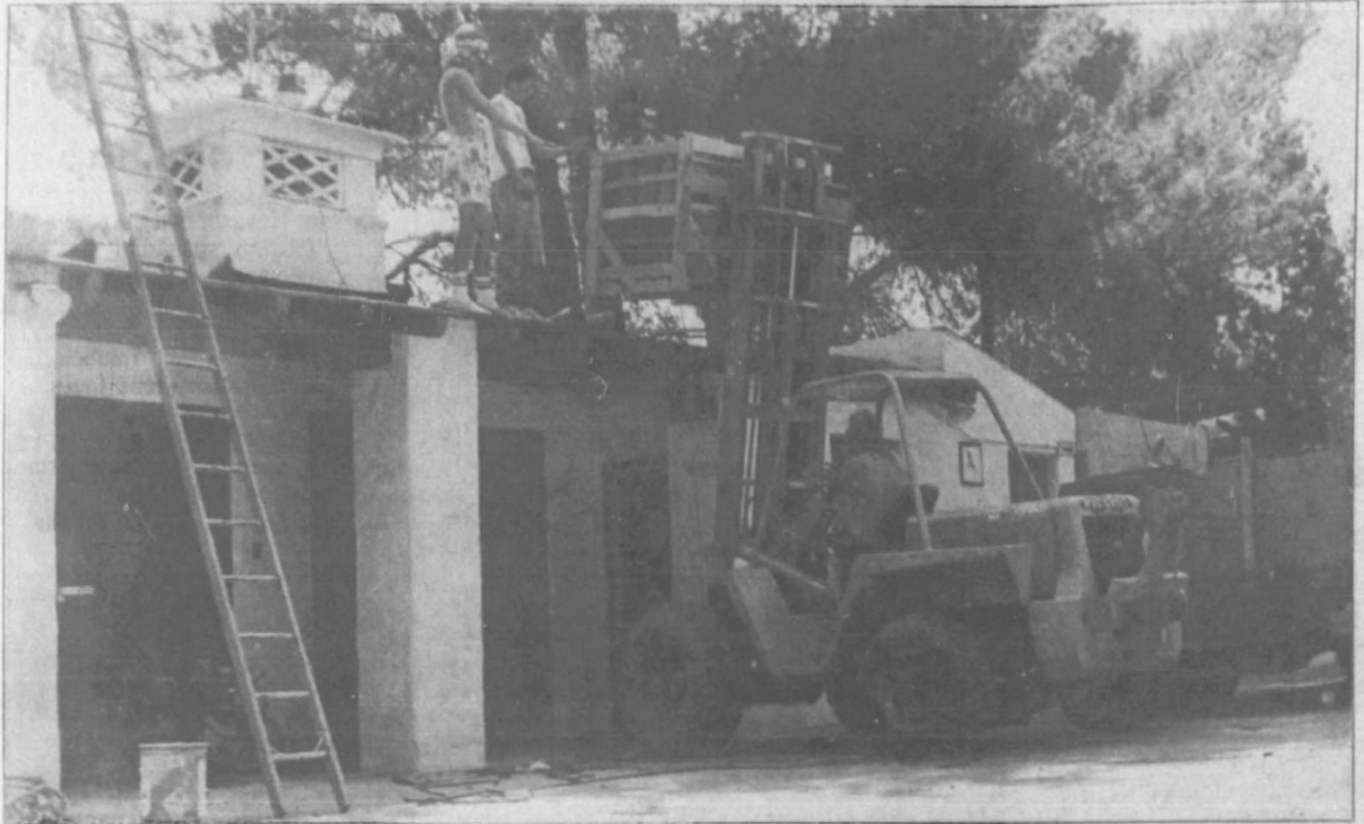
Workers, above, deliver clay tile for the roof of the Hart mansion. The original tile will be salvaged and reused
