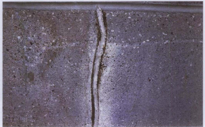
Figure 19. A high-speed grinder is used to widen a crack in preparation for installation of a sealant. This process is called "routing." After the crack is prepared, the sealant is installed to prevent moisture infiltration through the crack. Although sealant repairs can provide a durable, watertight repair for moving cracks, they tend to be very visible.
