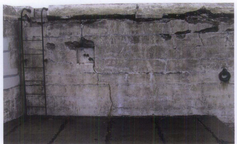
Figure 13. Fort Casey on Admiralty Head, Fort Casey, Washington, was constructed in 1898. The lift lines from placement of concrete are clearly visible on the exterior walls and characterize the finished appearance.
