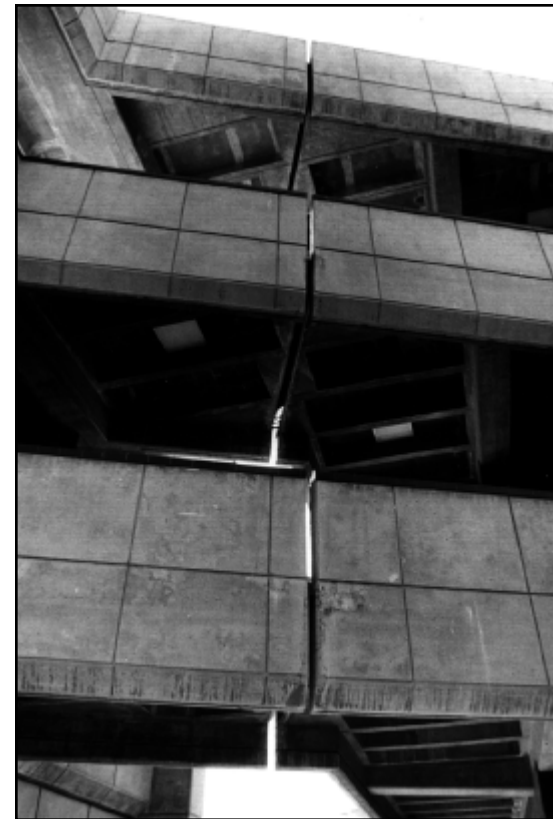
This expansion joint where the IRC (Bonelli Hall) and C Building (Seco Hall) meet was widened from the force of the 1994 quake.
