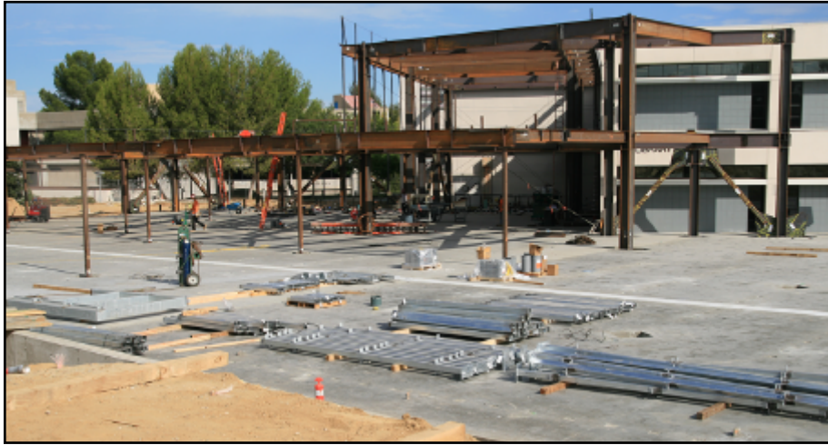
Construction begins to expand the library and create a new home for the TLC.
