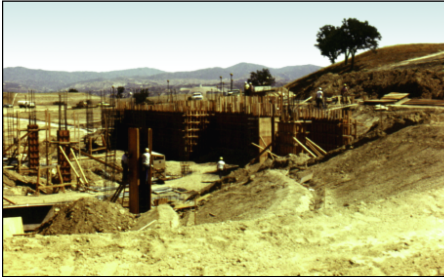
Construction workers build the forms that will encase the massive poured-concrete foundation of the Instructional Resource Center (Bonelli Hall).
