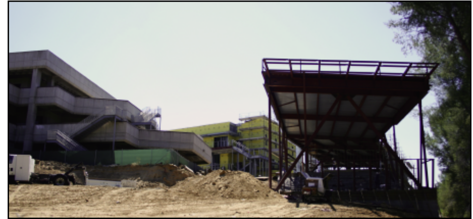
Construction of Aliso Hall (above, right) and Aliso Labs (above, center) moves forward adjacent to Boykin Hall (above, left) in mid-2006.
