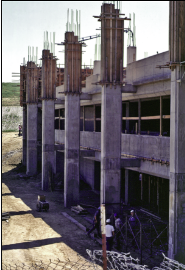
The Instructional Resource Center (Bonelli Hall) begins to take shape, having risen two of its eventual four stories.
