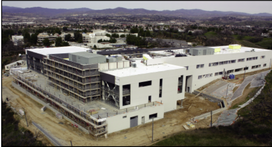
The University Center takes shape in this low-aerial view looking northeast in February 2009.
