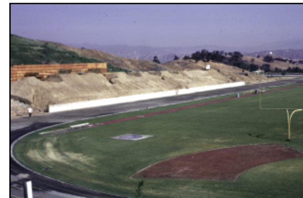
A crane hoists a bank of lights into place at Cougar Stadium, which itself is under construction (top). An earlier photo (above) shows the field, running track and a mound of dirt that was used as the foundation for the stadium.
