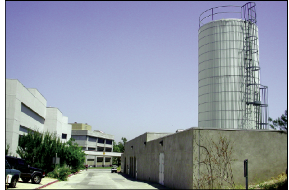
The Central Plant (above) was built to provide heating and air conditioning to two new buildings: the Media & Fine Arts Building (now called Mentry Hall) and the Library. Its efficiency resulted in a 25 percent savings in energy costs.
