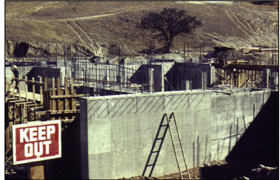
The foundation of the IRC (Bonelli Hall) begins to take shape on the College of the Canyons campus.
