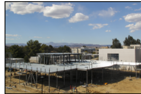
Chancellor Dr. Dianne G. Van Hook (top) speaks during the groundbreaking ceremony for the culinary arts facility, which was soon under construction (above).
